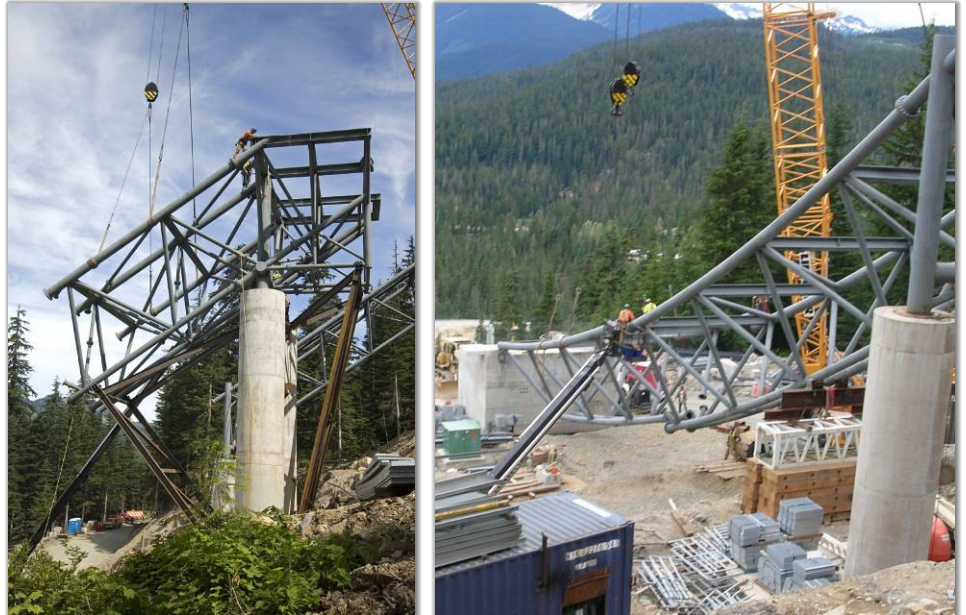
carefully planned shoring was used to meet the precise erection tolerances for this structure
